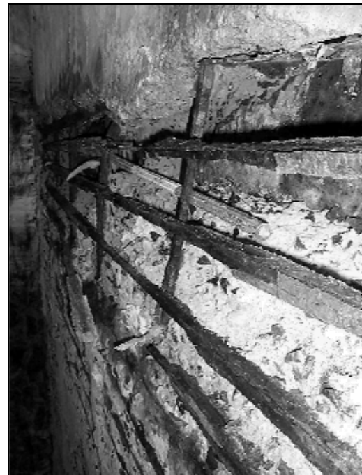
Exhibit IV. 3 Severely Deteriorated Reinforced Concrete
