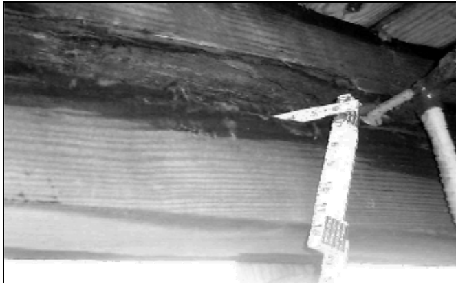
Exhibit IV. 1 Severely decayed timber beam
